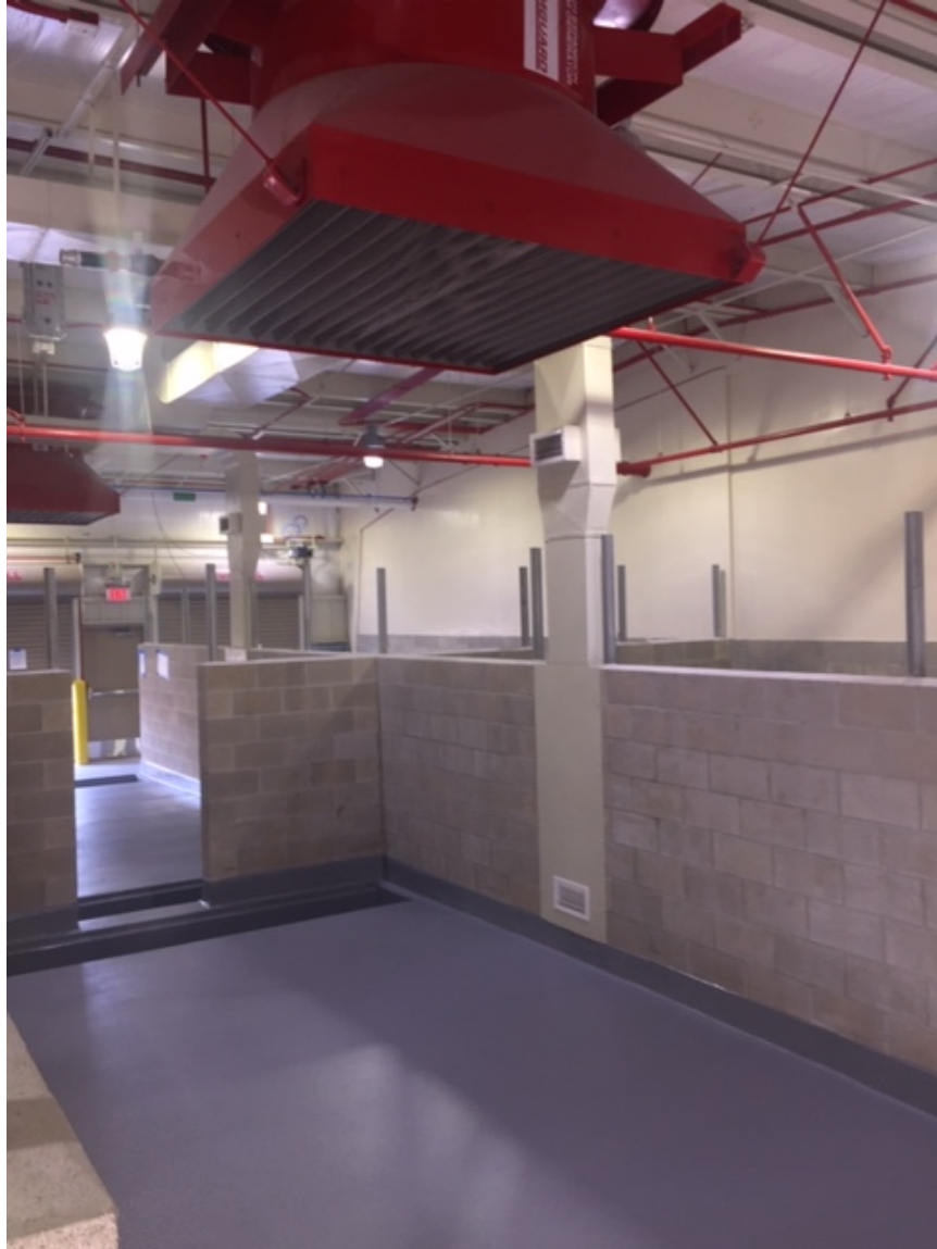
Hazardous waste storage bay fire foam system.
