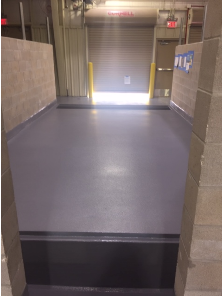
Hazardous waste storage bay and secondary containment and grating.
