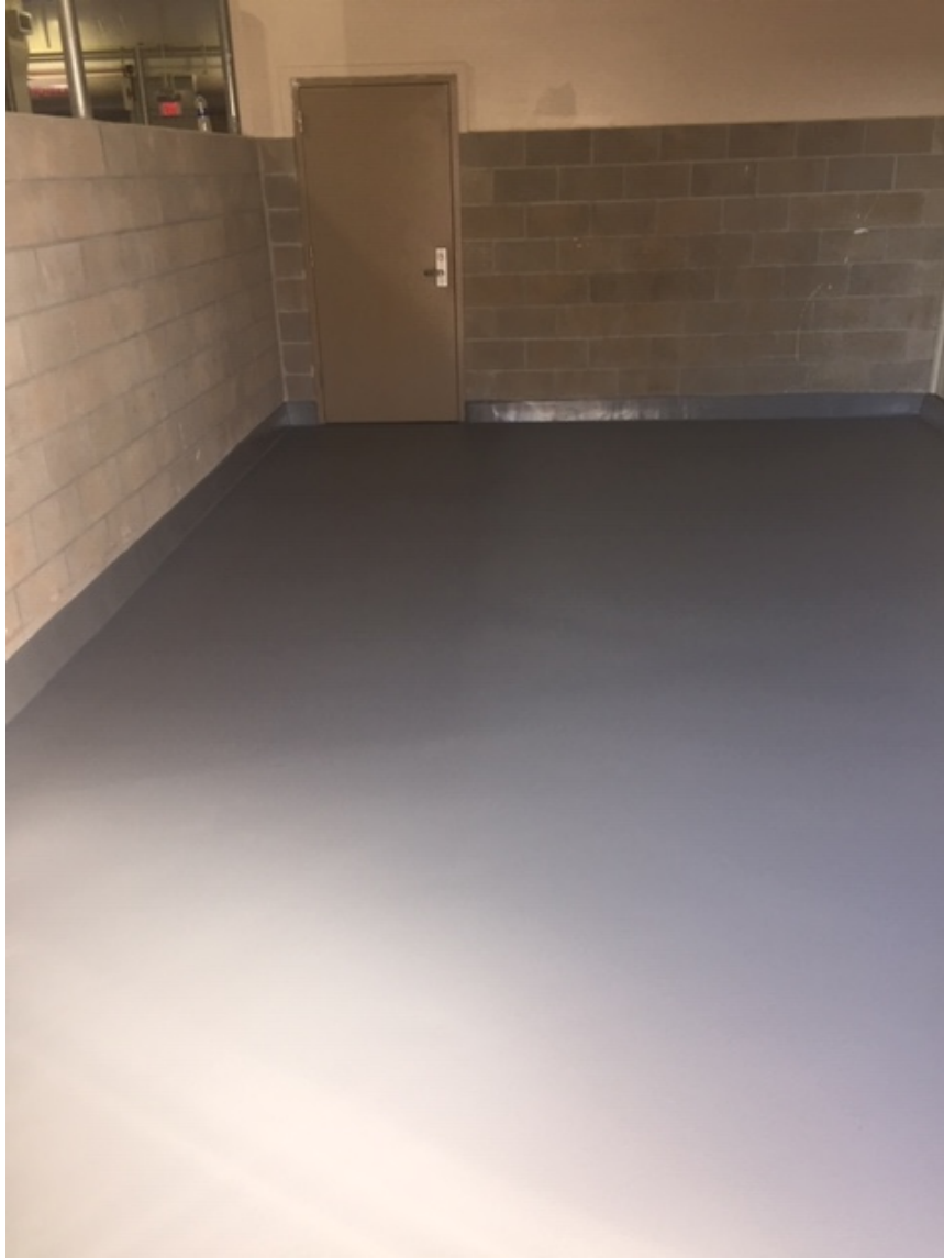
Equipment and materials storage bay.
